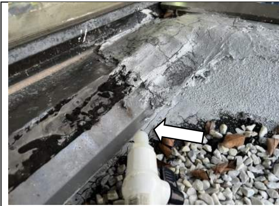
Image 65, Negative Pressure – View of smoke infiltration testing in progress at the exterior. Note: Smoke observed at interior when applied to base of flashing beneath lead-coated copper sill flashing.
