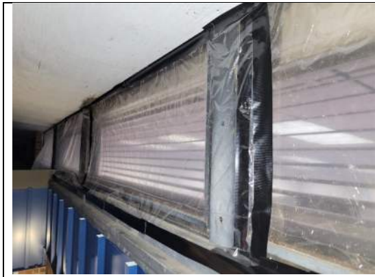
Image 83 – Plastic sheeting was install to provide temporary isolation to suspected air leakage source paths.
