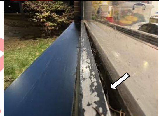
Image 14 – View of missing glazing gasketing.
