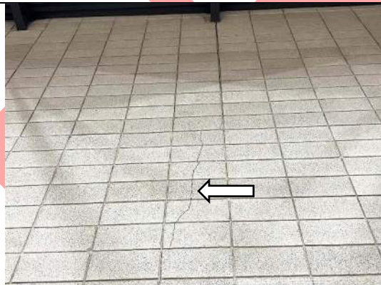
Image 19 – View of step cracking crossing both mortar joints and masonry units. Similar cracks were observed at other faces of interior walls in gymnasium.
