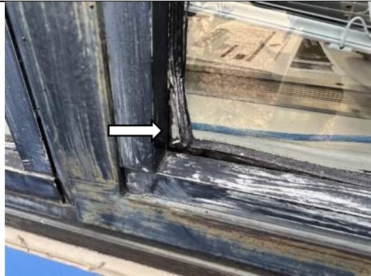
Image 13 – Representative view of failed window glazing gasket at Room S, the Nurse’s Office.
