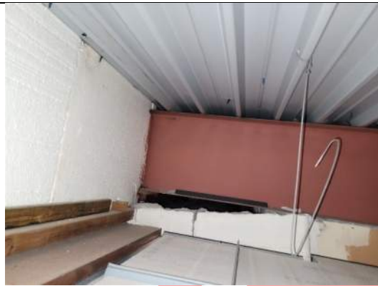
Image 29 – A partial view of the roof-to-wall transition above the clerestory windows within the ceiling plenum of a Pod-style classroom. Note, the gap between the steel beam and the top of the infill wall, and EPS insulation installed at the roof-to-wall transition.
