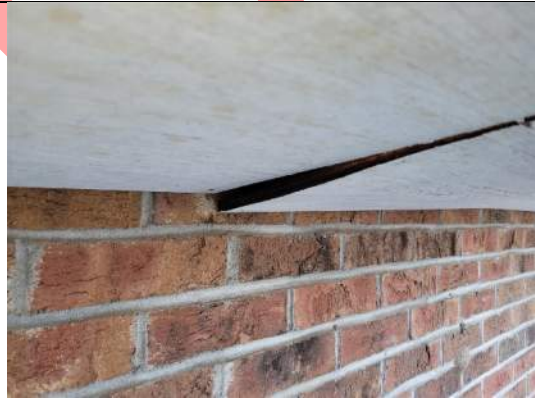
Image 5 – View of dislodged plywood soffit.
