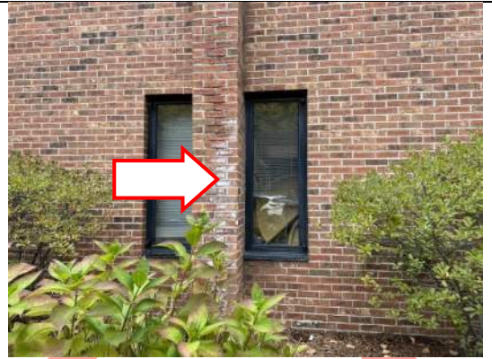
Image 2 – Atmospheric staining and efflorescence observed on face brick pier, located at the exterior side of the office space between Rooms D and C.
