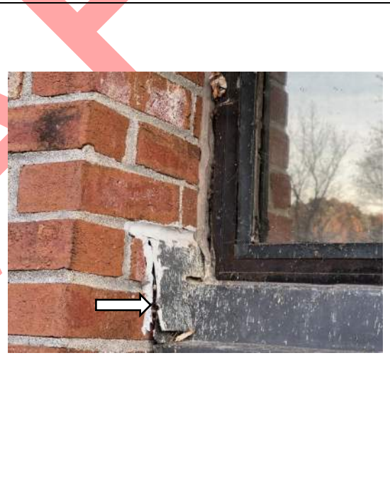
Image 10 – View of displaced flashing and failed sealants located at the exterior side of Room 26.
