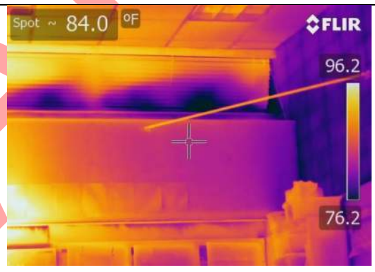
Image 68, Negative – Evidence of air infiltration observed at the sill of the clerestory windows.
