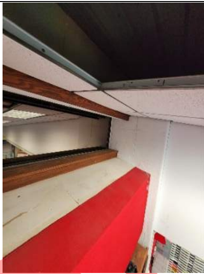
Image 85 – Partial view of the area within Room 7 where access to the pier wall and soffit condition were attained.
