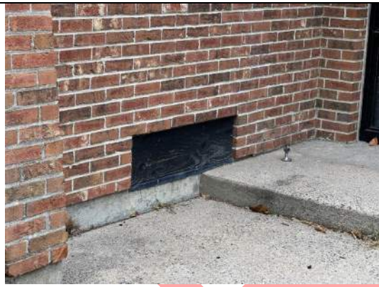
Image 3 – View of plywood infill where existing louvers were noted to be present located adjacent to the entrance to Room C.
