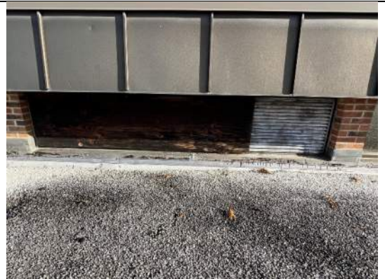
Image 6 – View of plywood sheet over existing louver at the exterior side of Room 7.
