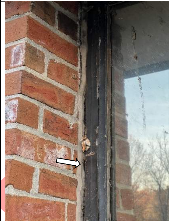
Image 9 – View of deteriorating perimeter sealant located at the exterior side of Room 26.
