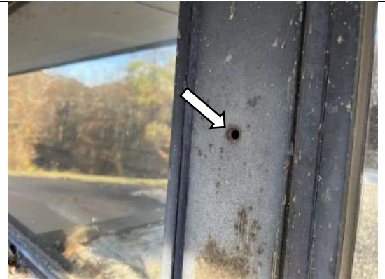
Image 8 – View of missing fastener at vertical mullion between clerestory windows. Condition observed at several locations.
