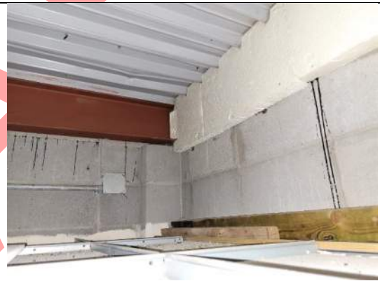
Image 30 – A partial view of the roof-to-wall transition within the ceiling plenum of a typical classroom. Note, EPS insulation at the roof-to-wall transition.
