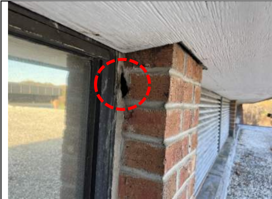
Image 7 – Hole in brick pier between clerestory and louver, indicated by red dashed circle.
