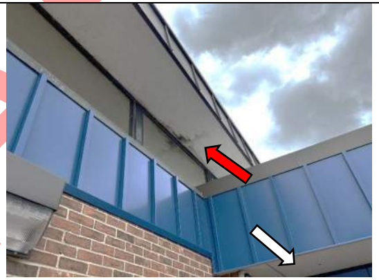
Image 4 – View of stained plywood sheets at clerestory soffit (red arrow), a condition generally observed at clerestory windows. Note: Similar looking Glasweld panels used in original construction (white arrow).
