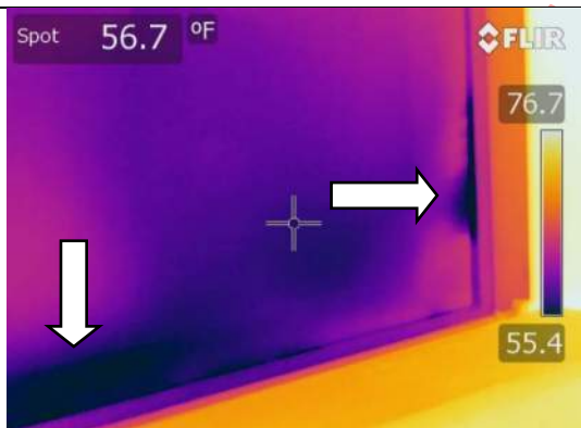
Image 67, Negative – Evidence of air infiltration observed at the jamb of the window sash.
