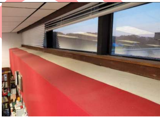
Image 69 – Interior view of the bulkhead located beneath the clerestory windows in the Pod Classrooms.
