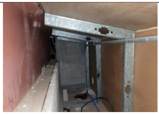
Image 70 – View of the partially exposed masonry pier wall from within the bulkhead. Unsealed gaps between construction elements can provide a path for air movement through the exterior wall assembly.
