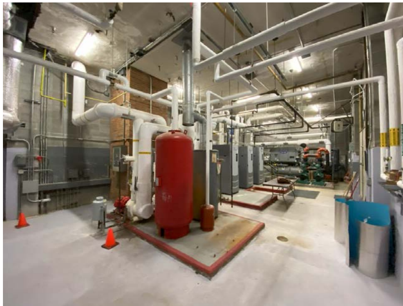
Boiler & Chiller plant feeding 2-pipe system
