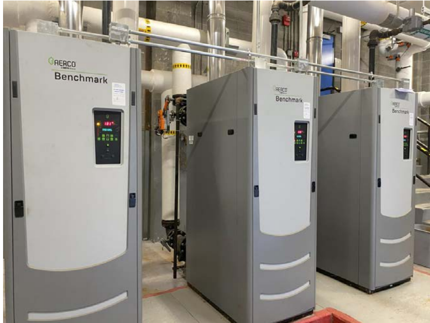
Condensing boilers - recently replaced
