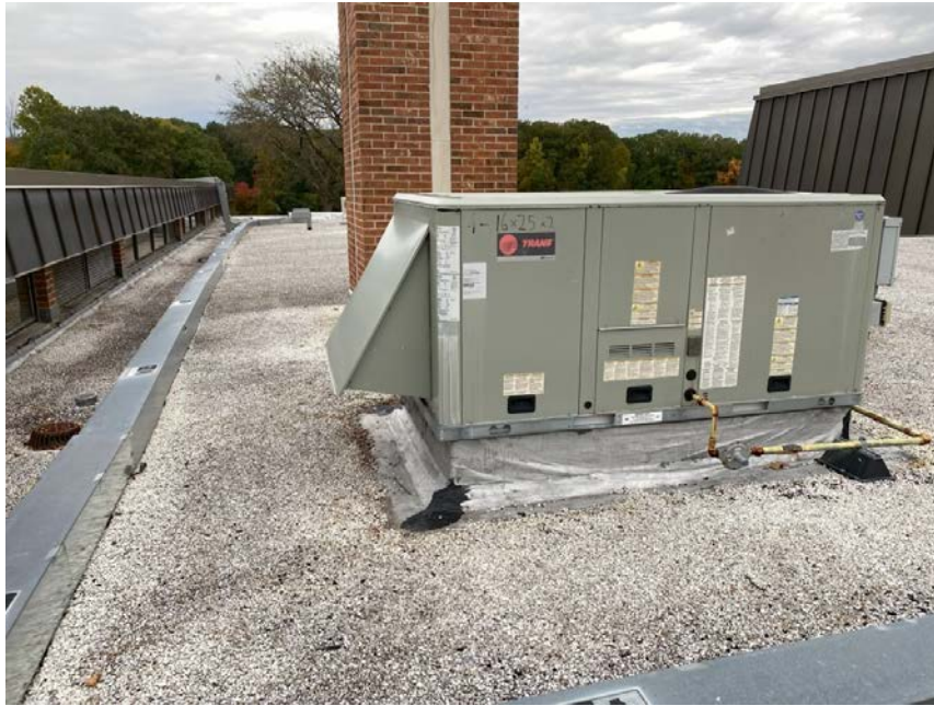
Packaged rooftop unit serving Office area
