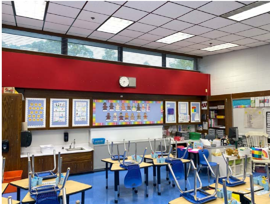
Typical Classroom showing Unit Ventilator
