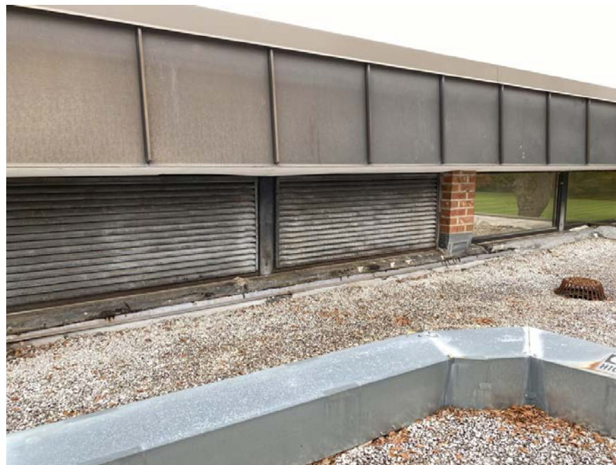
Typical fresh air lower serving Unit Ventilators
