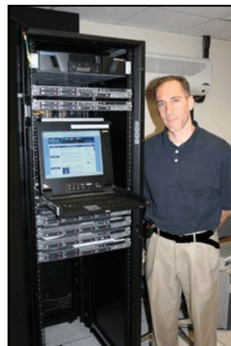
Frank Angelillo is pictured above in the town's main data center that services Local Area Networks used by town staff at offices in nine locations.
