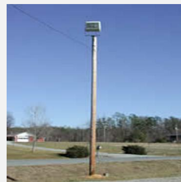
Utility Pole Floodlight
