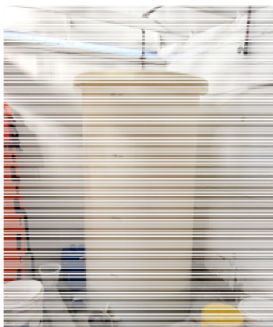
Chlorine Storage Tank
