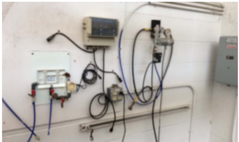
Abandoned Chemical Controllers
